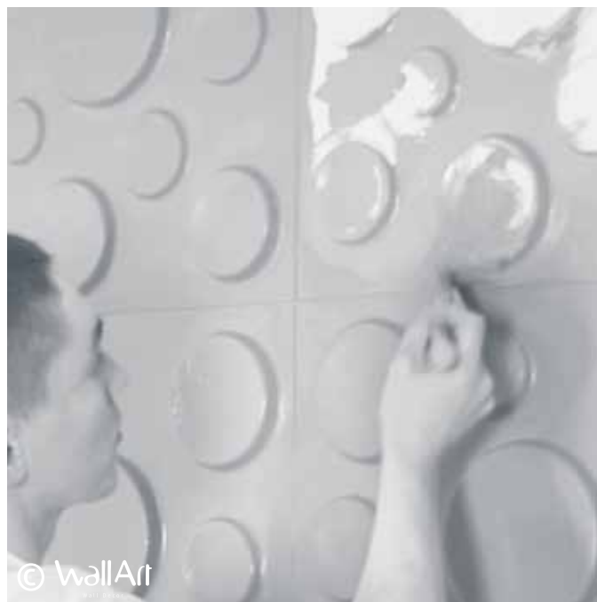
Paint Joints also
