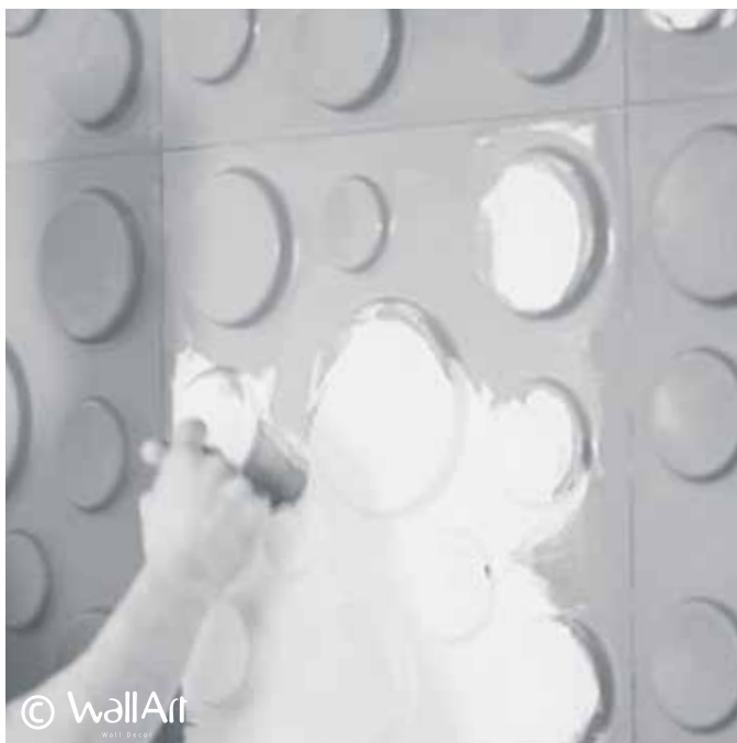
Paint without filling the Joints
